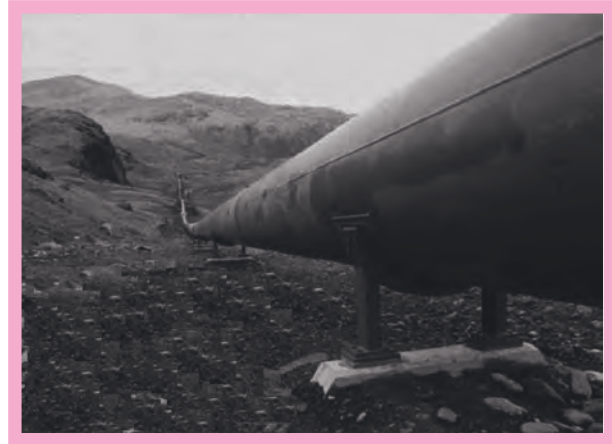
Non-Standard EasiSlide Bearings on Cym Dyli HEP Station, Gwynedd, Wales.
